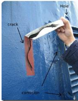
Duct tape and paint over a crack in funnel, Port State Control picture
